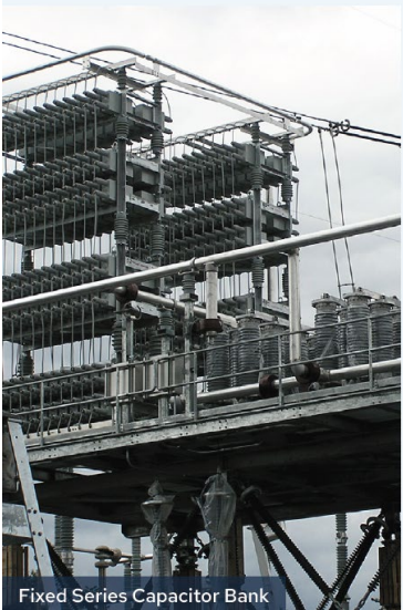
Fixed Series Capacitor Bank
