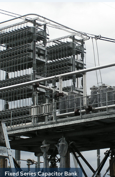
Fixed Series Capacitor Bank
